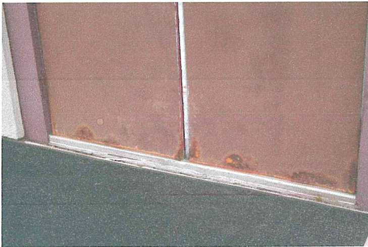
Pictured above top: Rear building entry doors Pictured bottom: Damage to door panels
