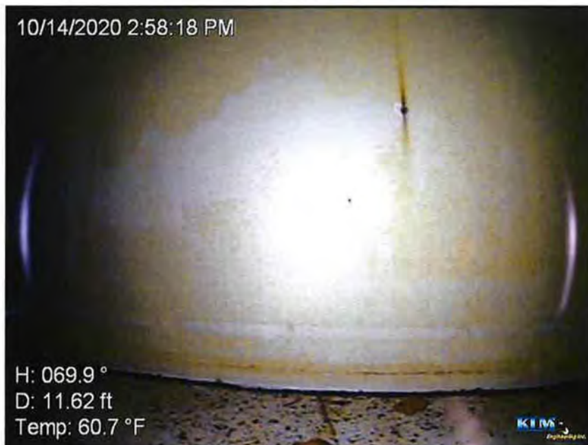
Photo No. 12 Lower shell condition
