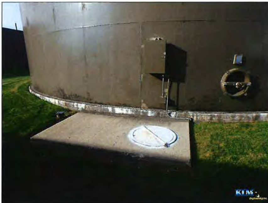
Photo No. 30 Shell condition, Note: cathodic protection equipment attached to tank
