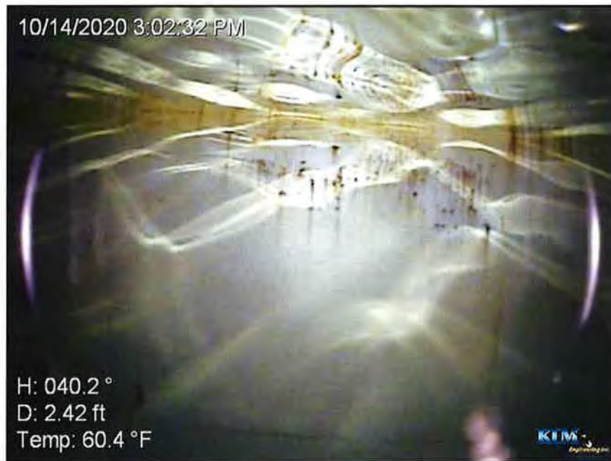
Photo No. 11 Coating failures on spot repairs on shell
