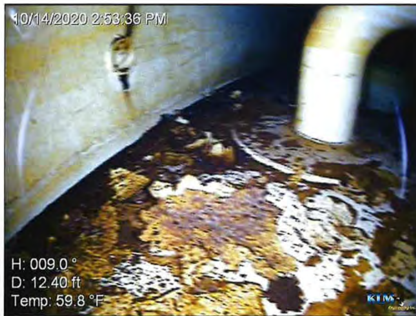
Photo No. 15 Paint chip accumulation on floor
