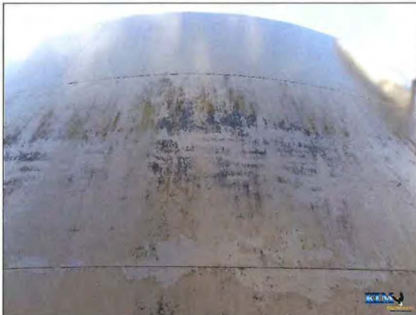
Photo No. 26 Condition of shell coating
