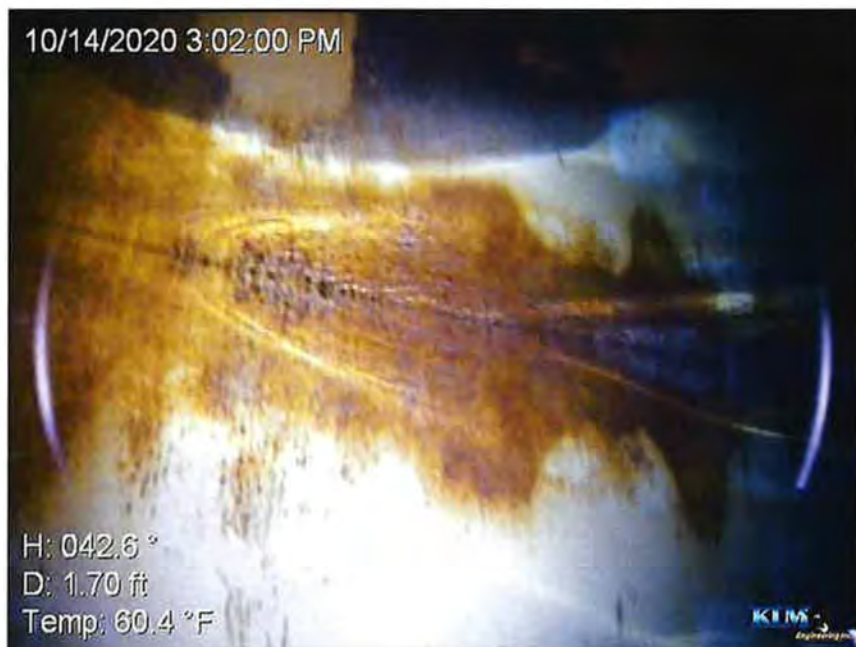
Photo No. 10 Condition of upper shell
