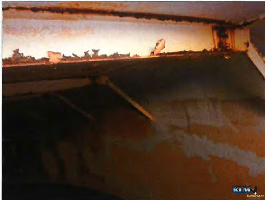
Photo No. 4 Severe corrosion on roof structure
