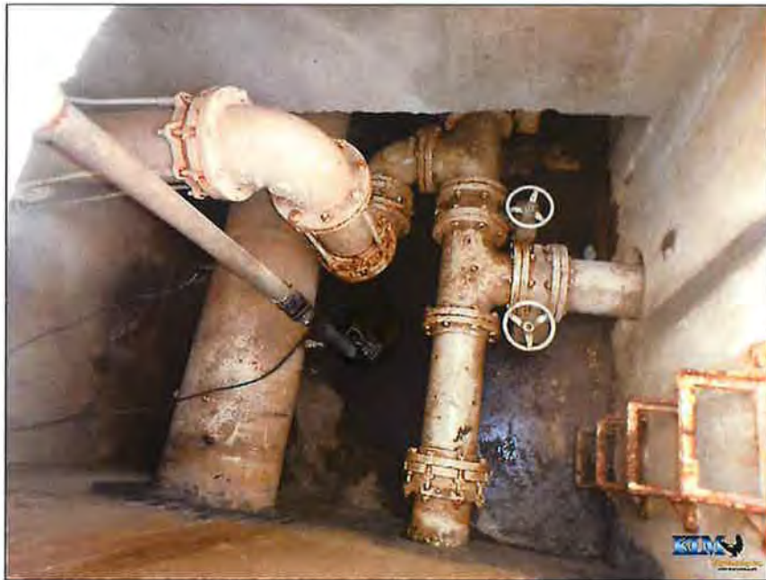
Photo No. 31 Piping in valve pit
