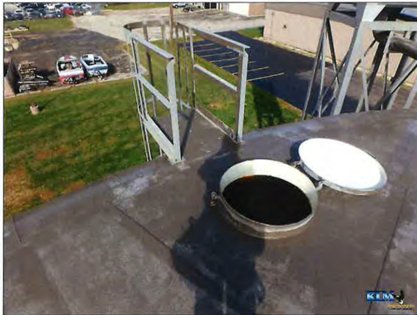
Photo No. 23 Access manway and ladder platform
