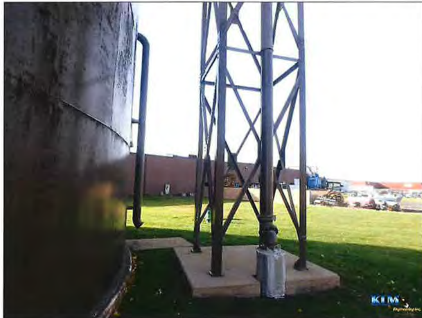
Photo No. 33 Abandoned aerator
