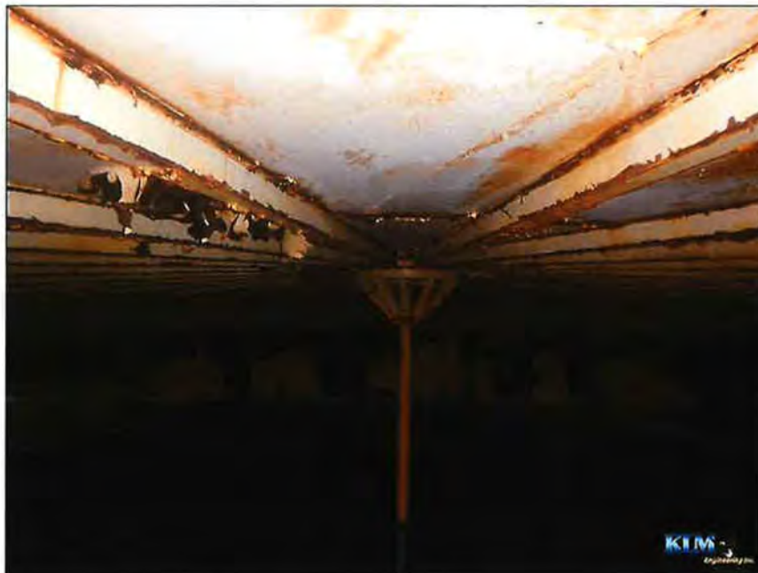
Photo No. 2 Center column and roof conditions
