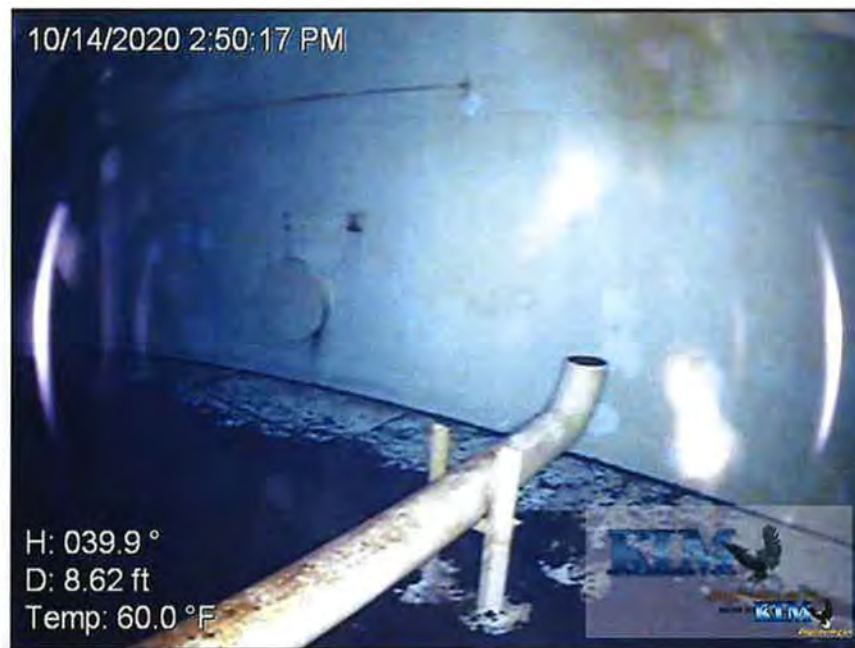
Photo No. 13 Lower shell/floor and fill pipe, Note: cathodic protection connection to shell
