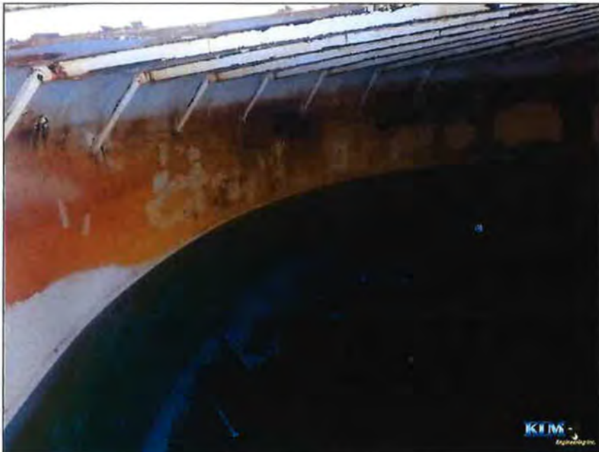
Photo No. 8 Upper shell condition
