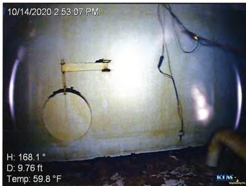
Photo No. 14 Shell manway and cathodic protection
