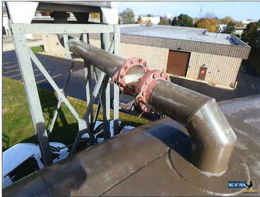
Photo No. 25 Abandoned aerator piping
