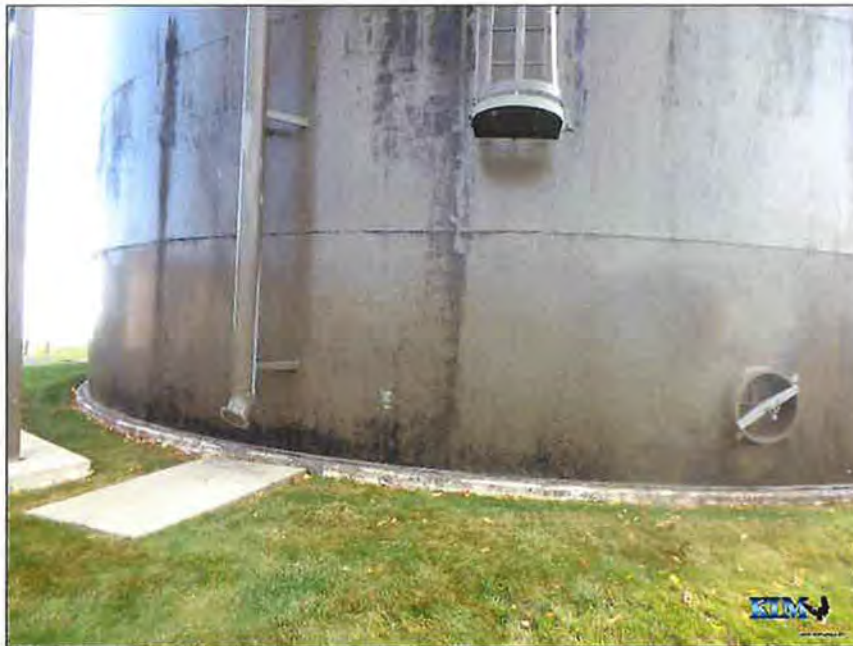
Photo No. 29 Shell coating condition
