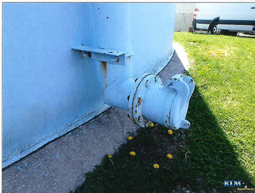
Photo No. 39 Overflow discharge, note missing flex cell at chime base
