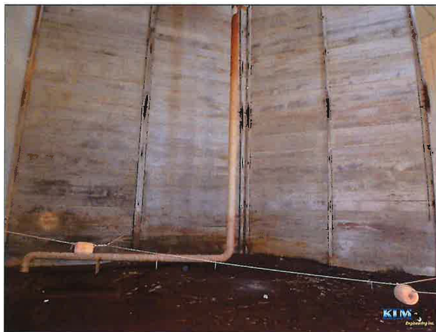
Photo No. 12 Fill pipe and baffle wall
