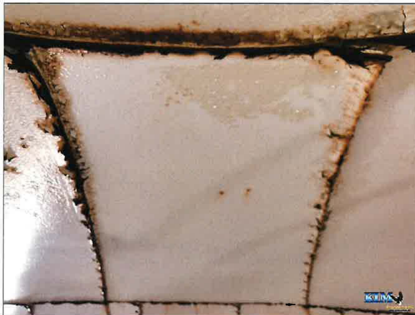
Photo No. 6 Severe corrosion on roof plates
