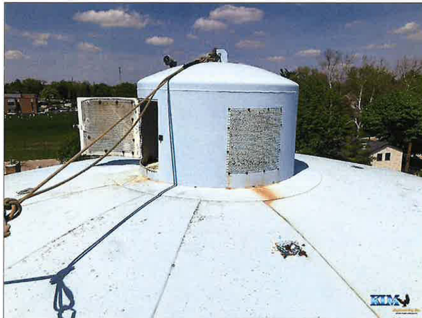
Photo No. 27 Non-compliant finial vent and roof conditions
