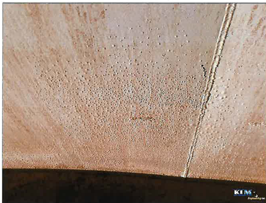
Photo No. 20 Shell coating condition, note blisters and erection scab marks
