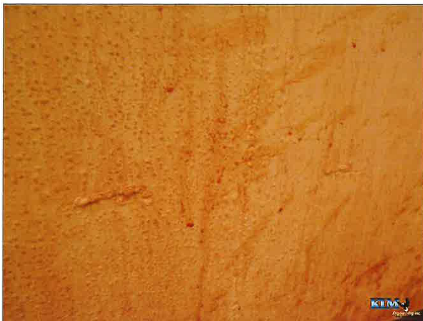
Photo No. 22 Erection scab marks and blistered coating on shell
