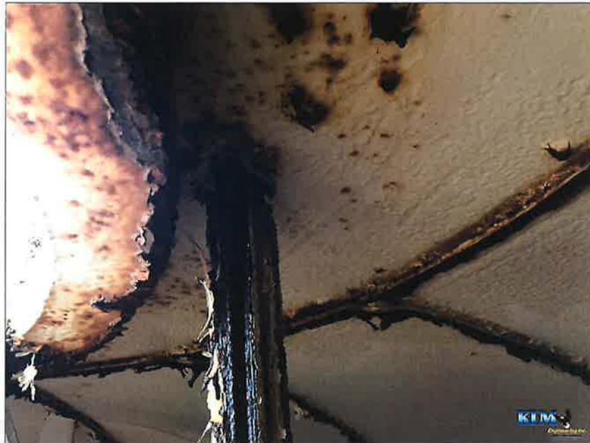
Photo No. 7 Severe corrosion on inspection platform brace and dollar plate
