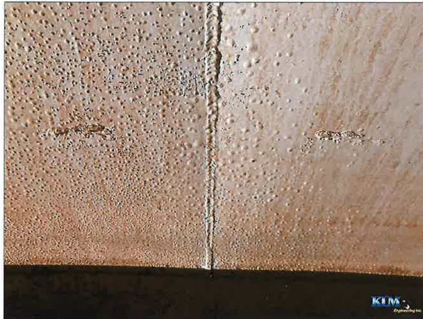
Photo No. 21 Erection scab marks and blistered coating on shell
