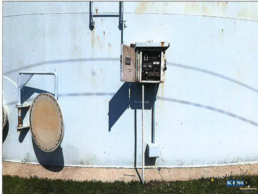
Photo No. 37 C.P. rectifier and shell conditions
