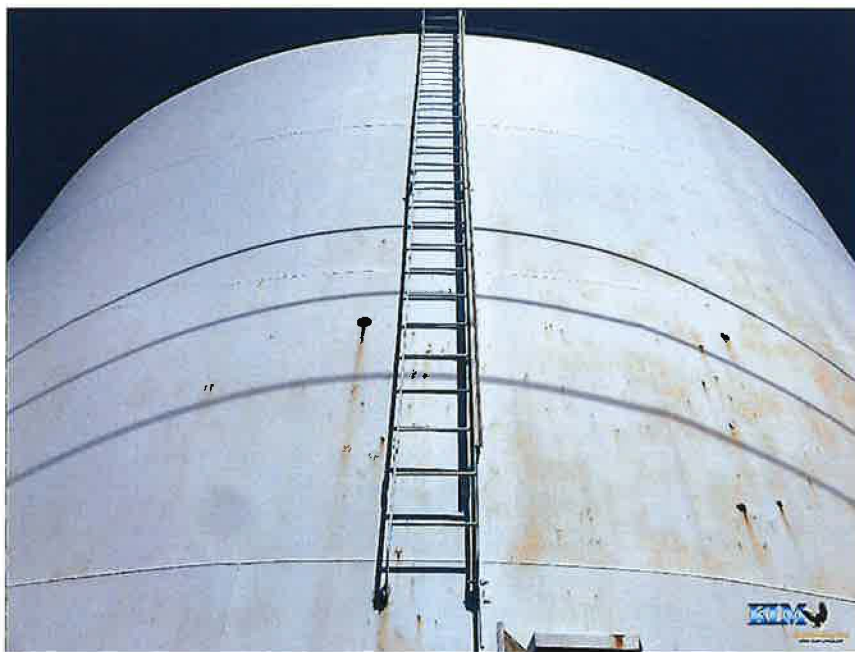
Photo No. 32 Shell ladder and coating conditions
