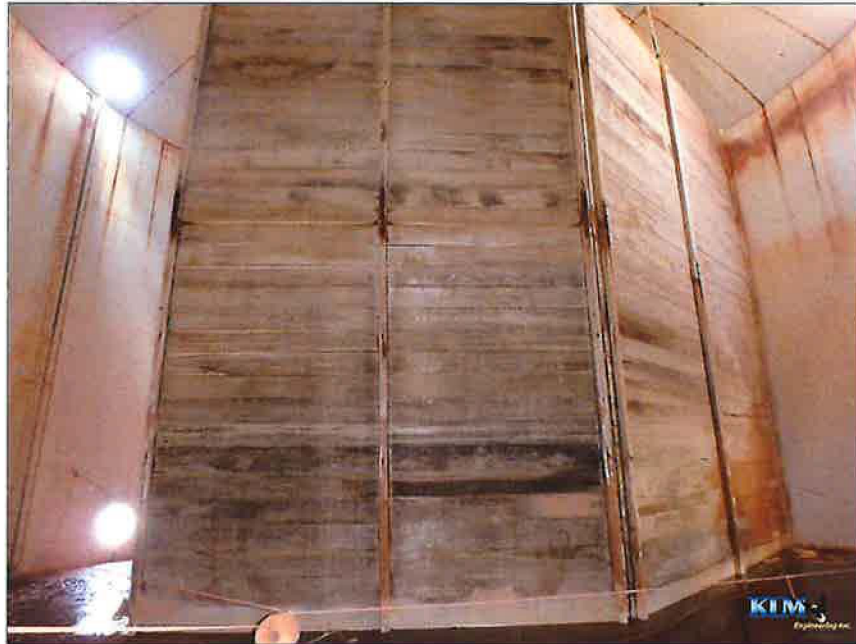
Photo No. 13 Wood plank baffle wall
