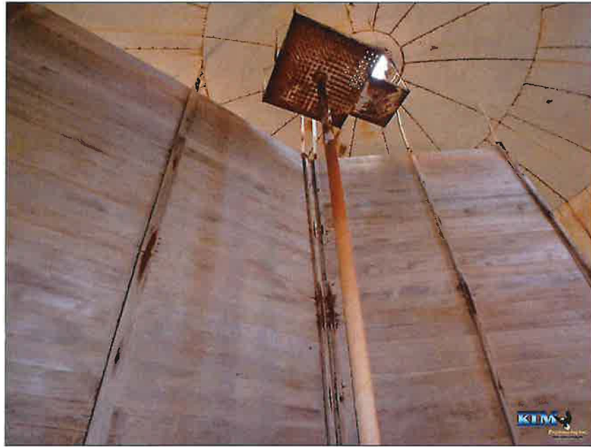
Photo No. 11 Fill pipe and baffle wall
