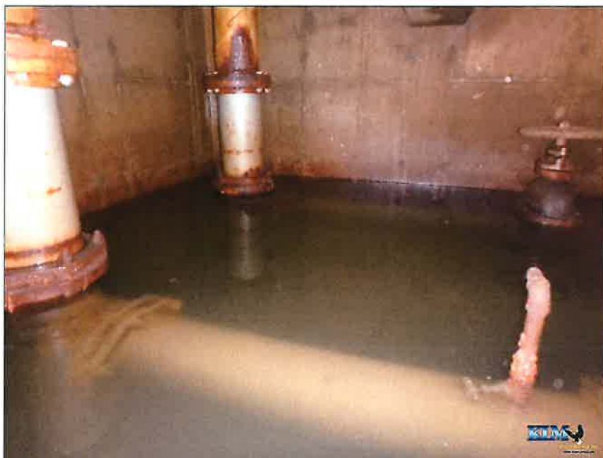
Photo No. 42 Valve pit and piping conditions
