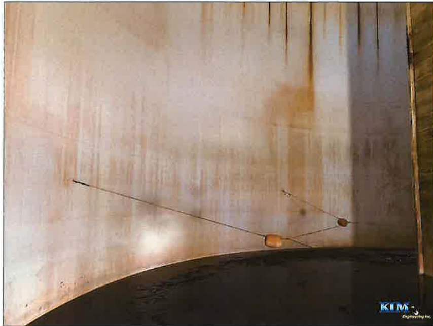
Photo No. 19 Shell condition, note C.P. system
