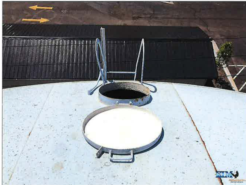
Photo No. 31 Note shell ladder location in reference to roof access manway
