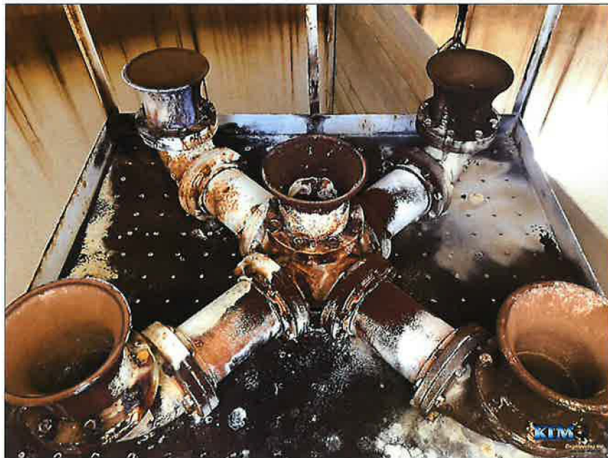
Photo No. 9 Fill pipe and de-fuser plate
