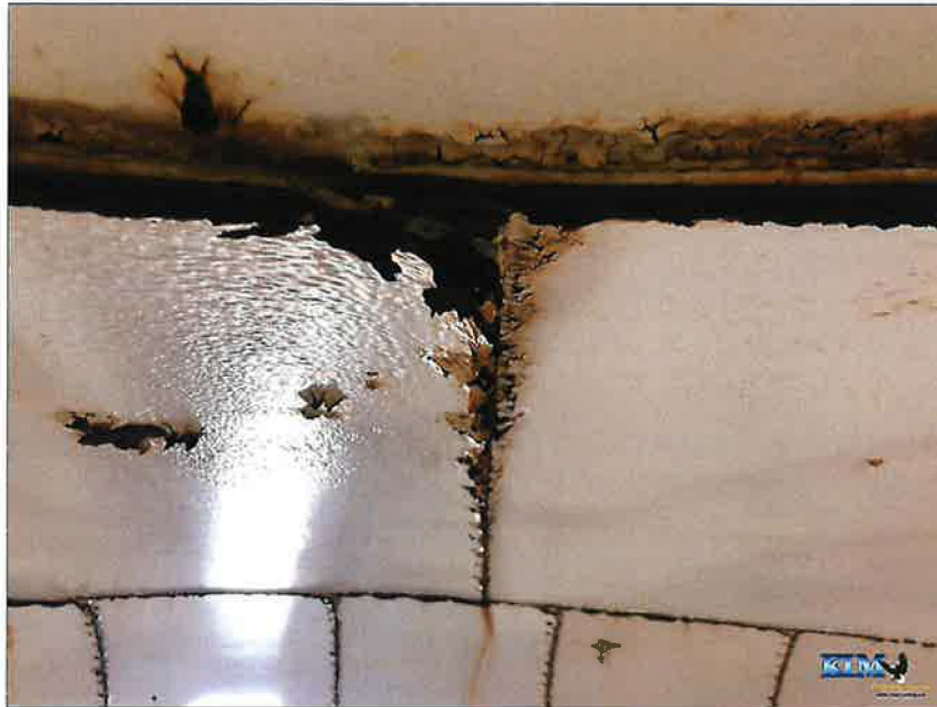
Photo No. 5 Severe corrosion on roof plates
