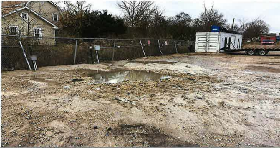
Taken 11/22/19 at 8:09 a.m. Site of Watermain Break 700 E Roosevelt Road. Water was throttled down at this time.
