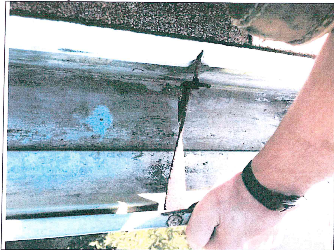
Hanger screw not attached to fascia.
